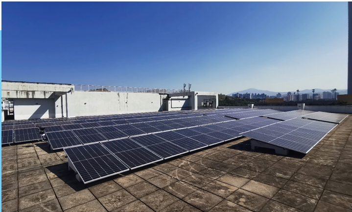
The solar power systems at Tin Shui Wai Exchange
